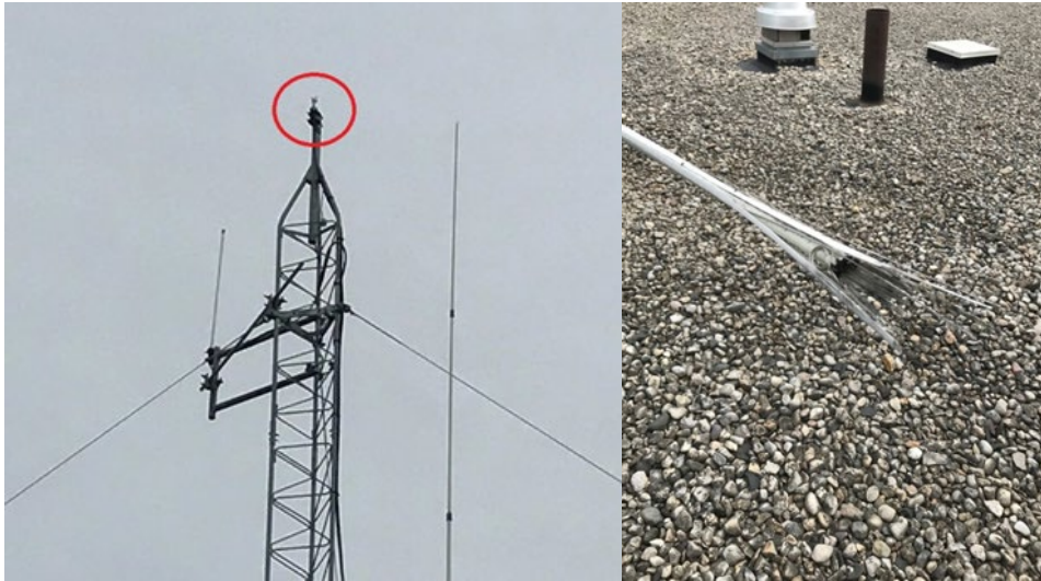
Figure 4.10.5: Two-Way Radio Antenna, hit by lightning, blown off the tower.
